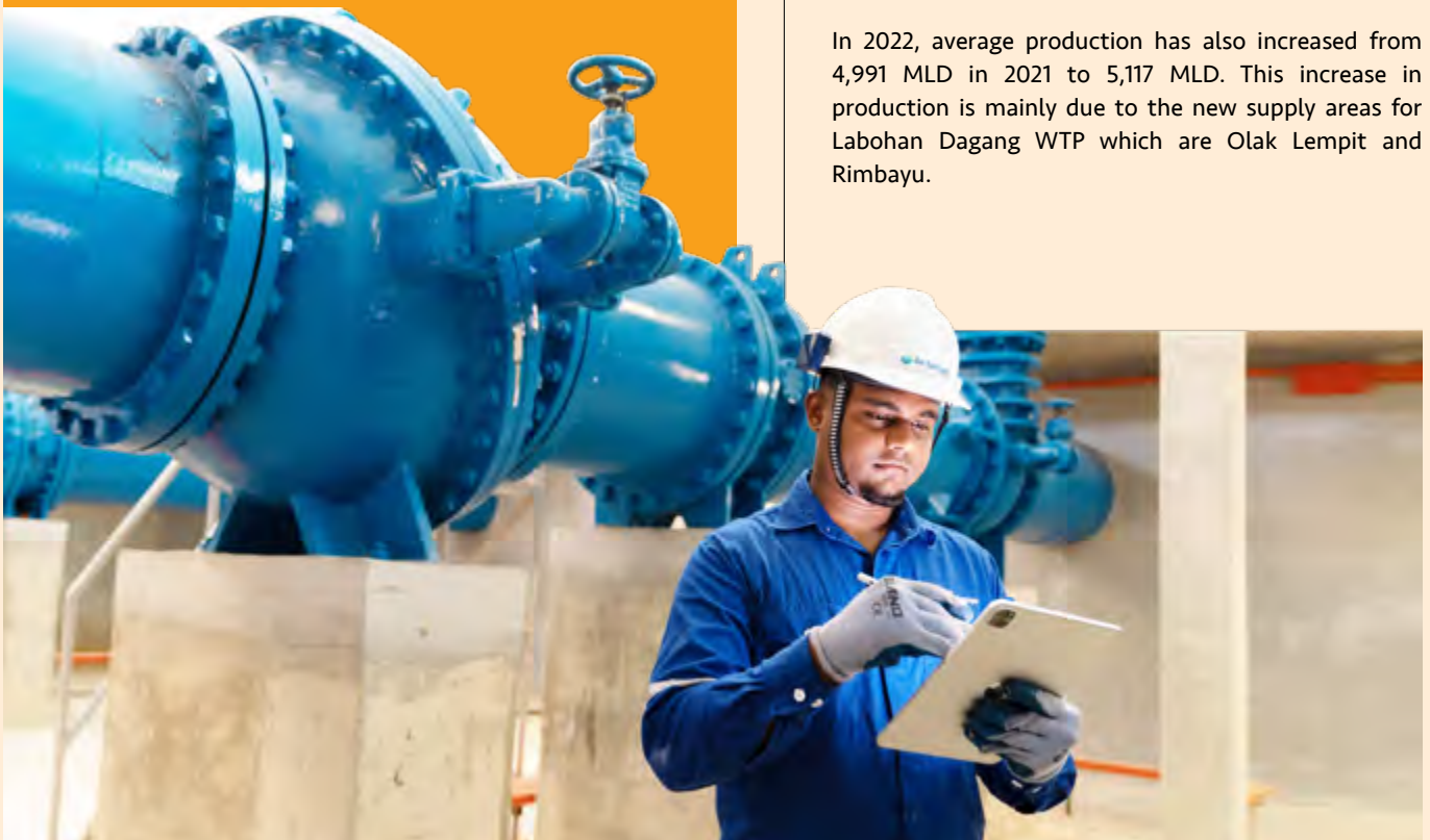
Pump House at Langat 2 Water Treatment Plant
