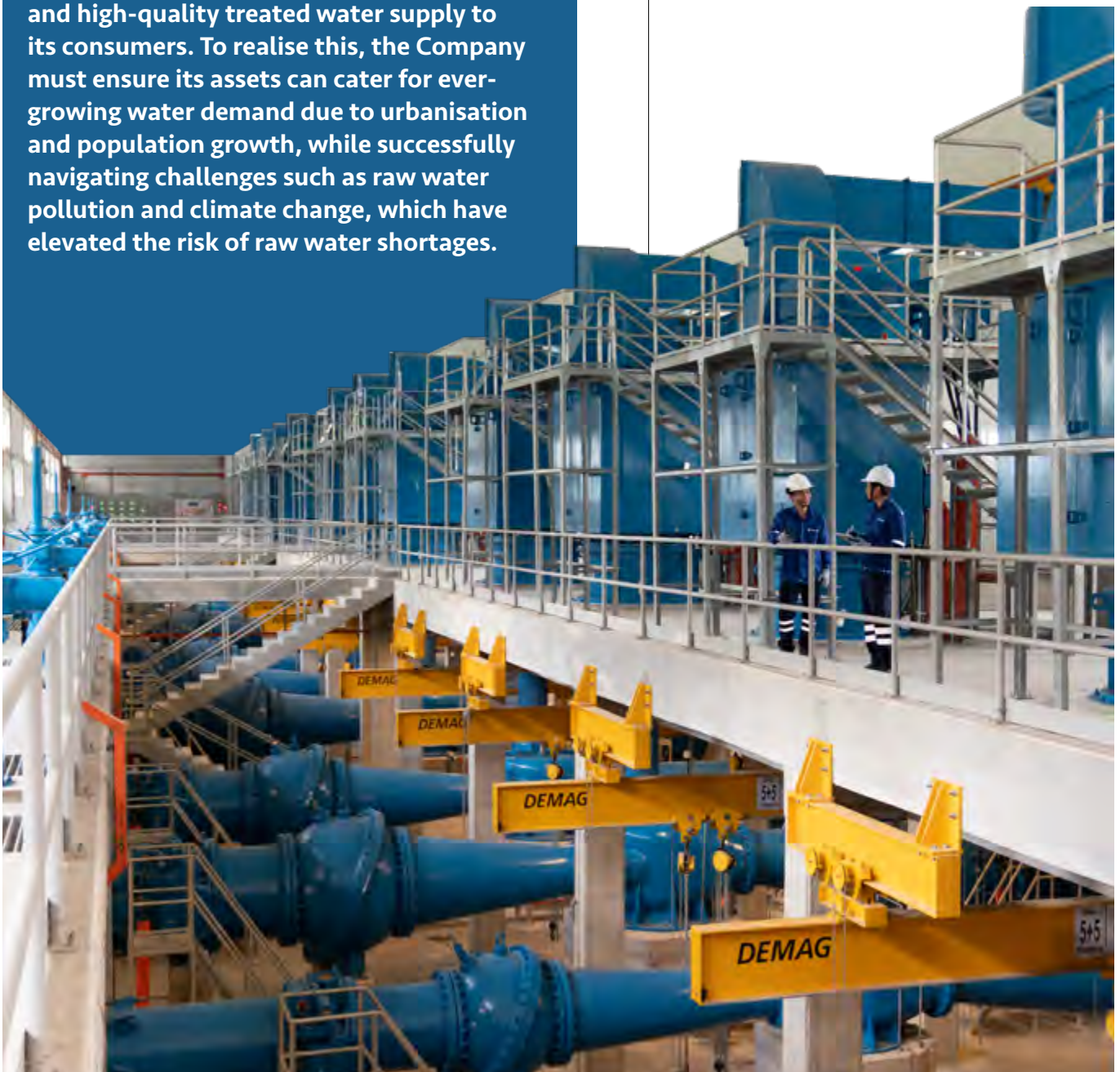
Pump House at Langkat 2 Water Treatment Plant
