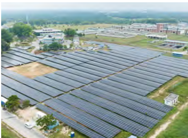
Solar Panels at Sungai Selangor Phase 2 (SSP2) Water Treatment Plant
