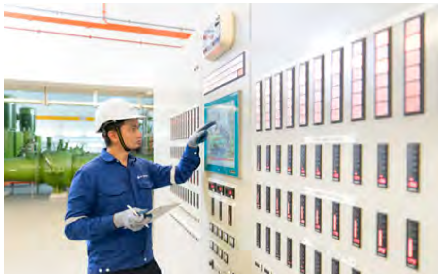
Control Panel at Filtration Tank Building, Langat 2 Water Treatment Plant
