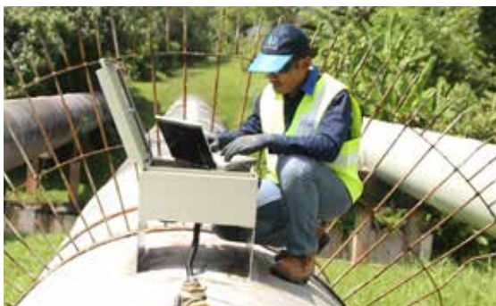
▶ Installation of 1,650 transient pressure sensors on main pipes to detect leaks much earlier, allowing repair work to be carried out immediately.
