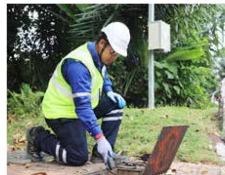
▶ The use of Permanent Leak Noise Correlating Logger to detect leaks in the reticulation pipe system. This online monitoring system allows immediate corrective action to be taken once a leak is detected in the pipe. As of December 2020, a total of 1,640 permanent leak detectors have been installed in 36 District Metering Zones.
